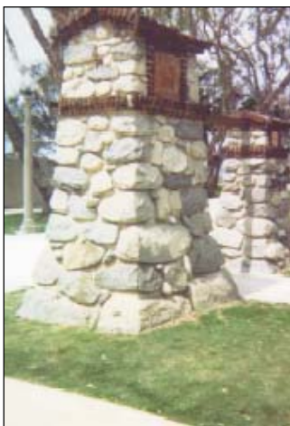
Example of a vertical gateway element made of stone and inscribed with a marker.
