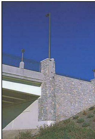
Example of decorative fencing and lighting treatments on a bridge. (Dublin, OH)
